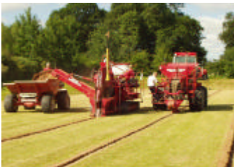
Sport England funded drainage work on the football pitches at Newton Farm
